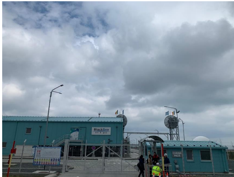
Image 3 Gas Treatment Plant in Vadu during site visit, April 2024
